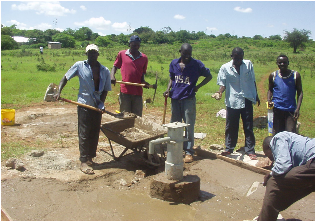
Villagers help install a hand pump at one of the Rotary water project sites In the village (Nyatike). “Oganga A well”
